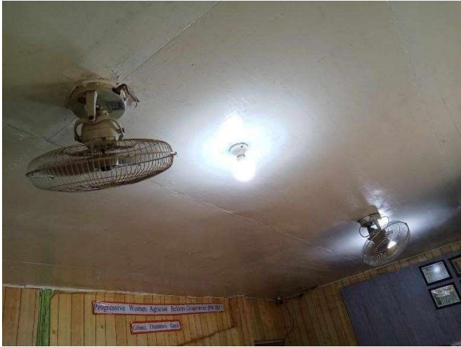
Use of LED lights and Fans instead of aircon
