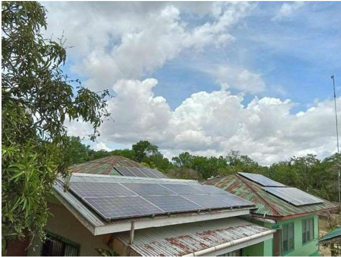
The Solar panels in the PWARC building & Processing Center
